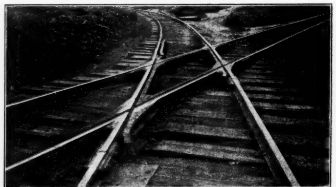
Fig. 5—Manganese Steel Crossing.
